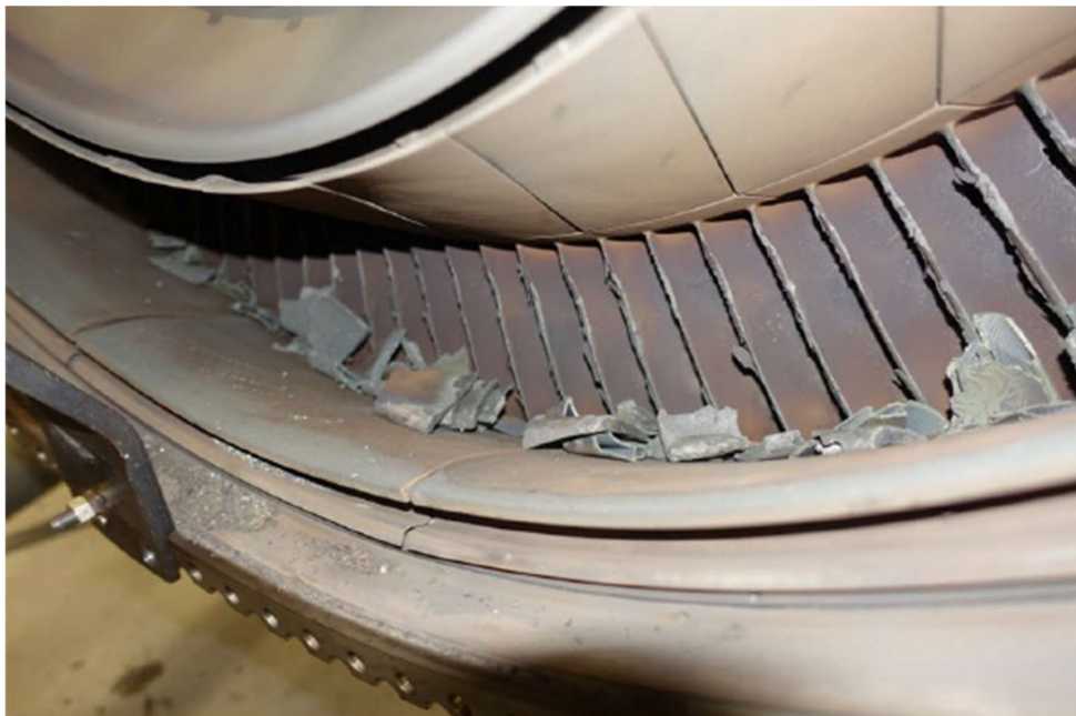
Metal Debris Accumulation on LPT Module Transition Liner
